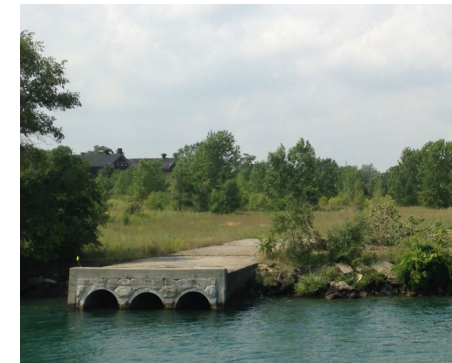
Combined Sewer Overflow pipes directed into the Detroit River 1
